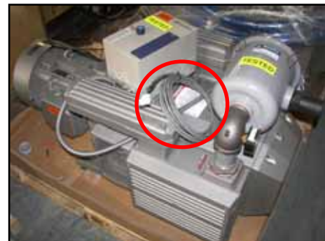
PICTURE 10: 3-Phase Wired Pump
