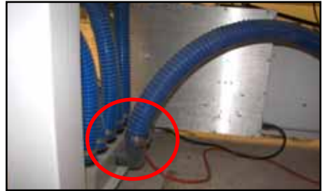
PICTURE 15: Manifold-Vacuum Hose Conn.
