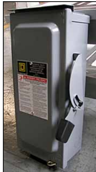
PICTURE 9: Power Disconnect Switch
